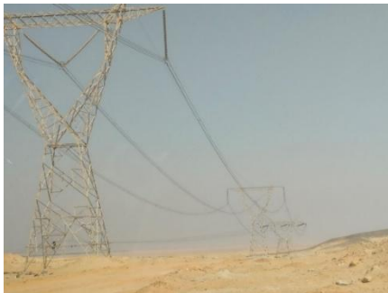
Figure 4-6: Overhead Transmission Lines in the proximity of project site
