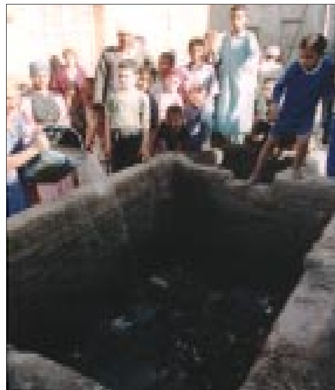
Grey water disposal tank
