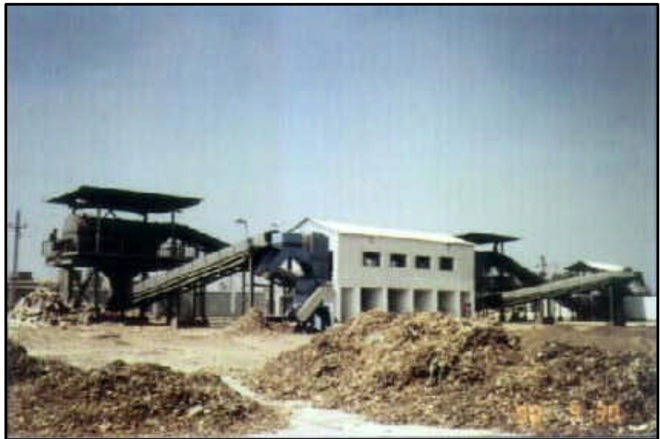
150 tpd Compost Plant Constructed for Mansoura City
