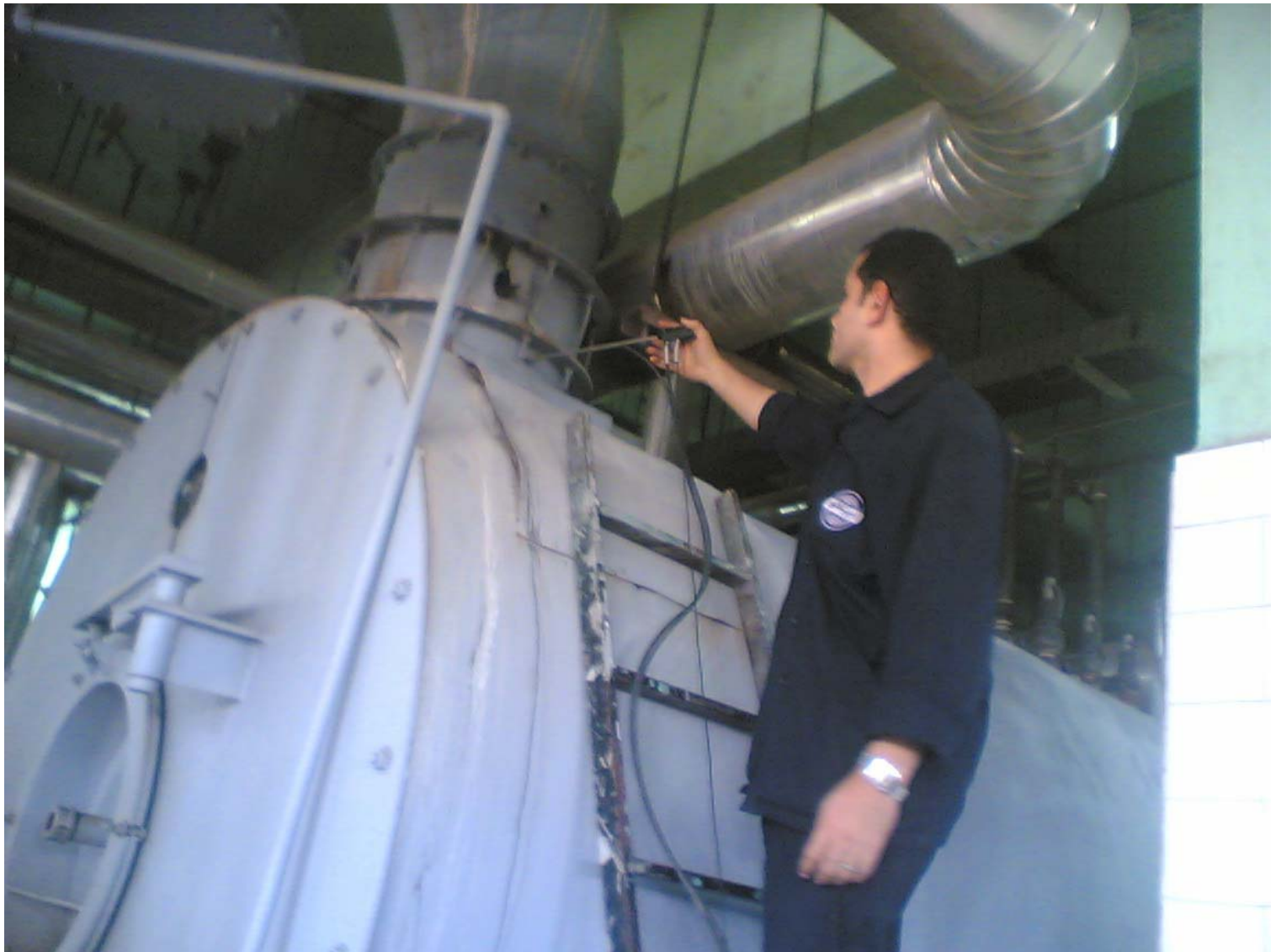
Measurement of air emissions from chimneys of a boiler
