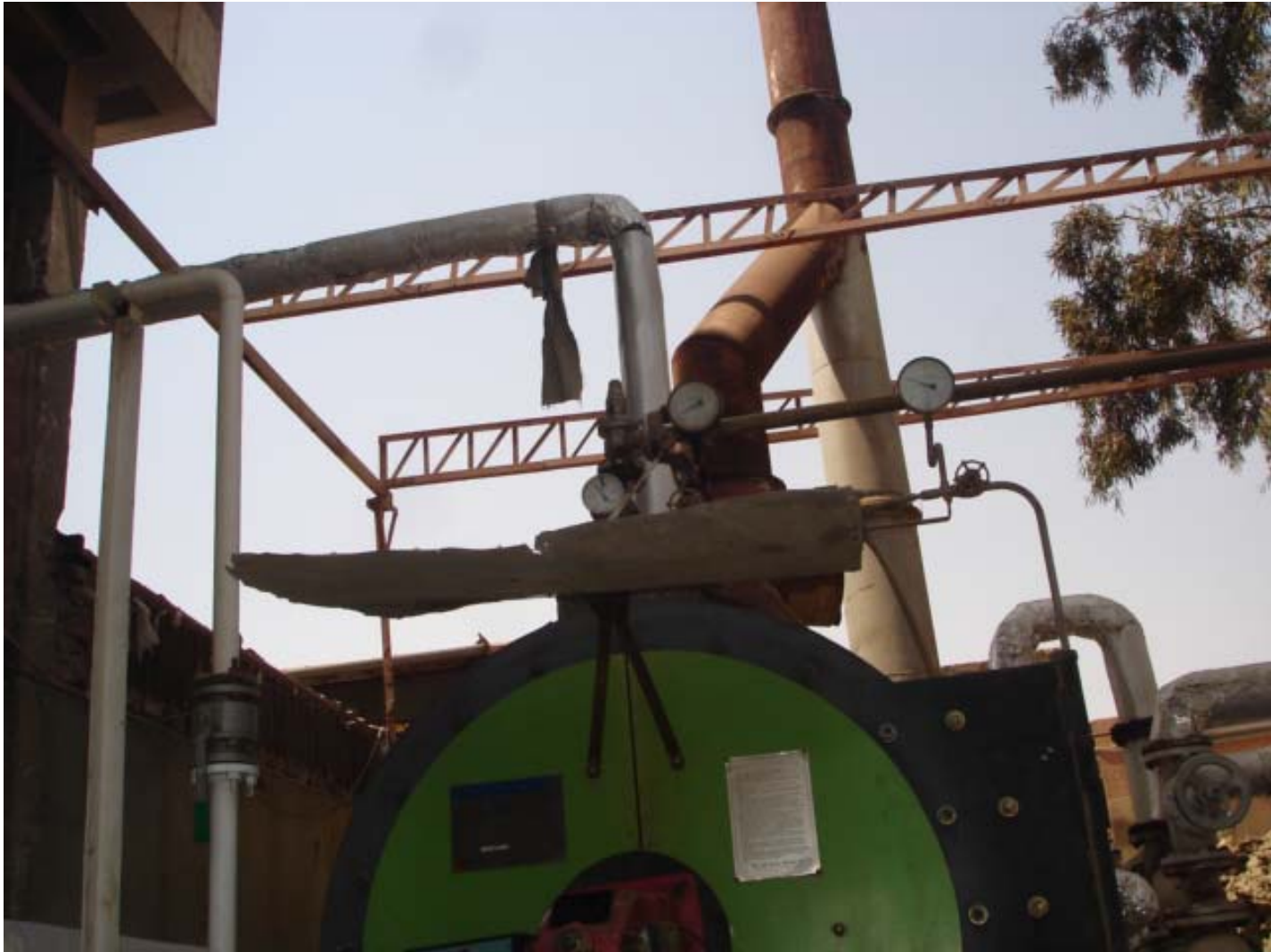
Main boiler chimney
