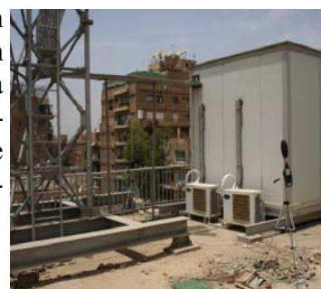
Picture (4-1) Noise measuring at mobile BTSs
